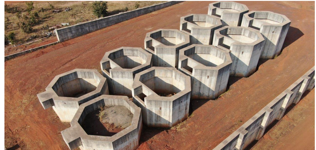
Rougher Flotation Cell Pedestals
