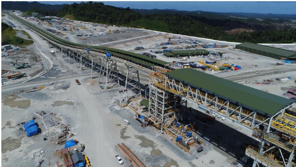
Figure 18-5 View of overland conveyors
