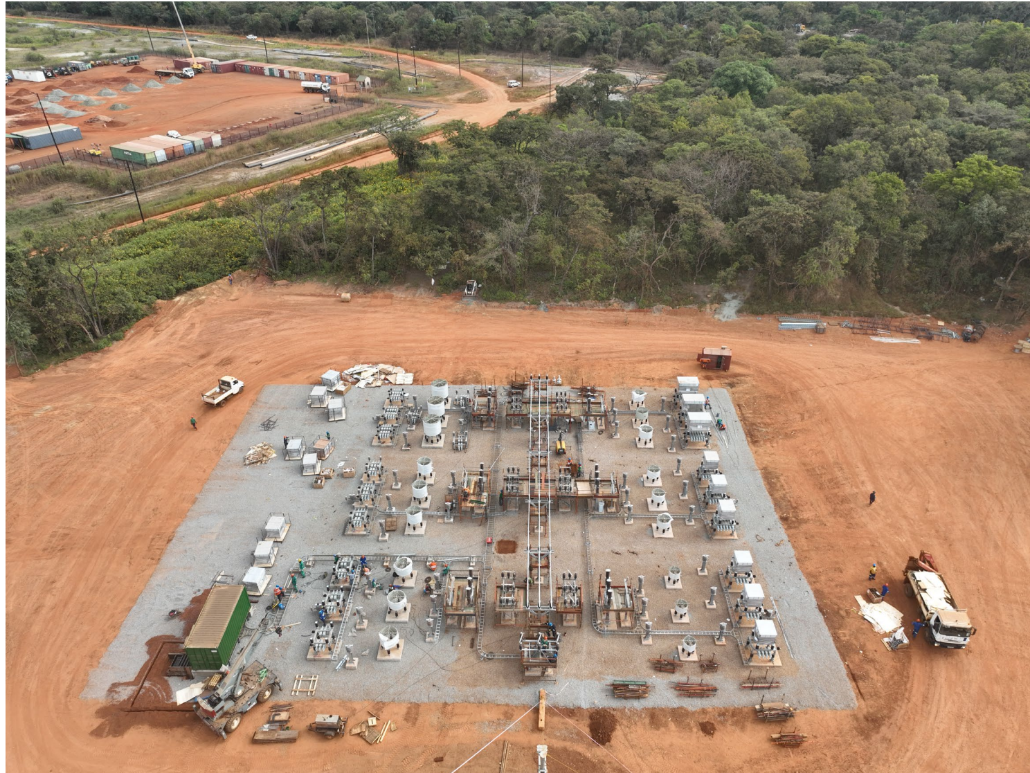
Power Factor Correction Yard
