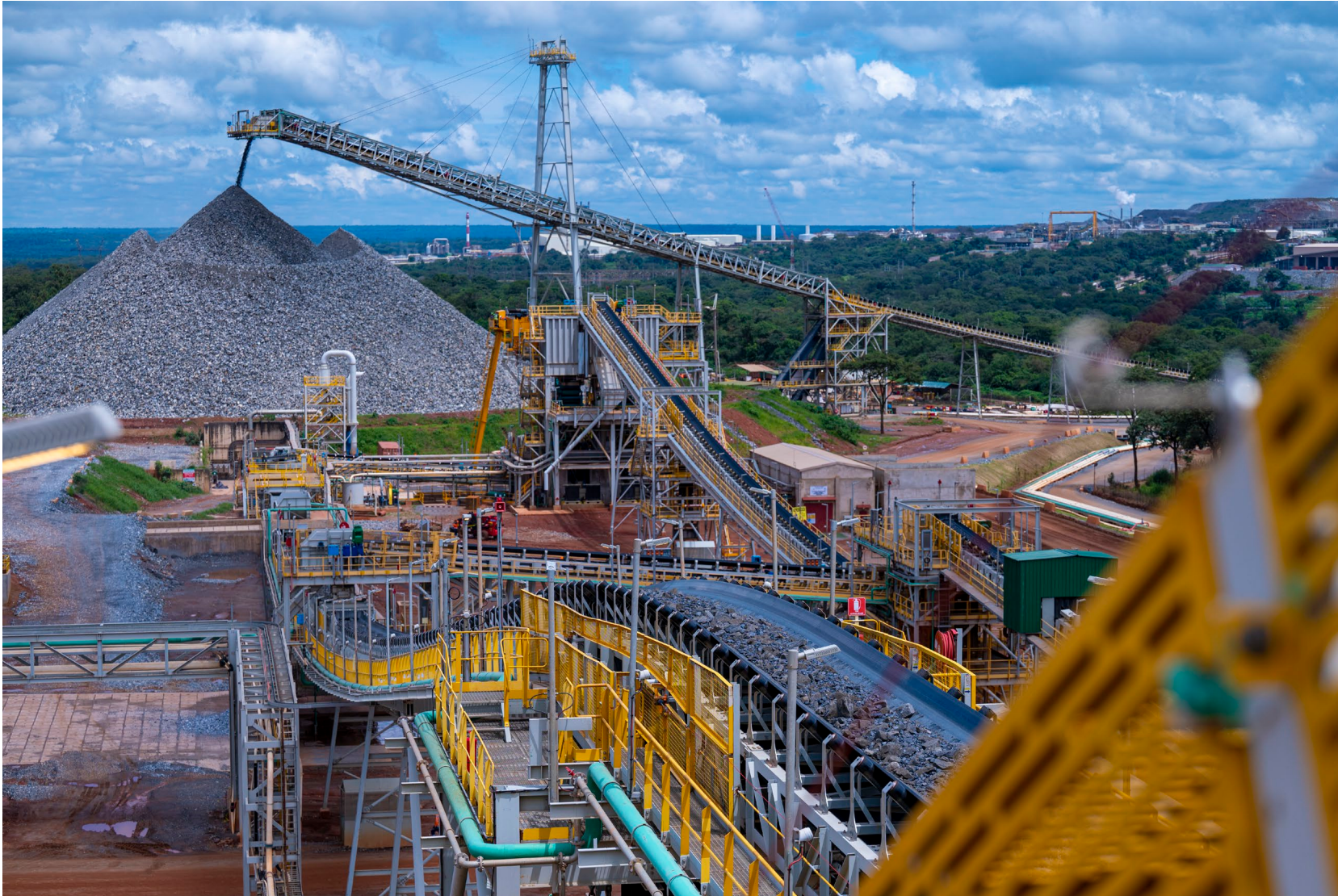
Stockpile Feed Conveyor
